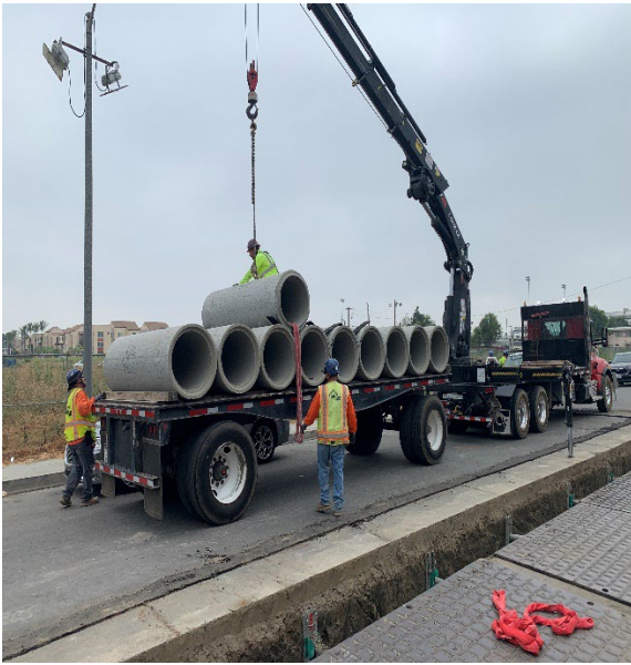
Area S4 – View of offsite storm drain June 5, 2024
