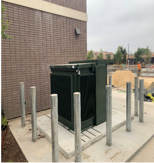
Area H2A - View of site electrical transformer June 13, 2024
