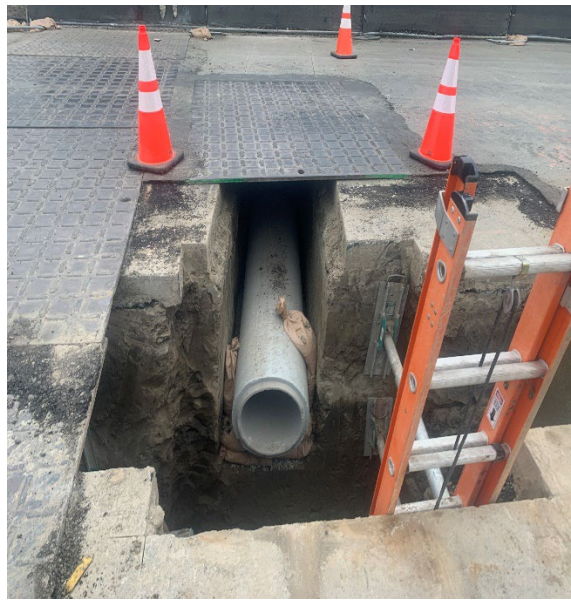
Area S4 – View of site offsite storm drain June 5, 2024
